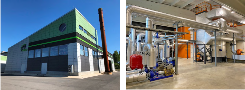
Figure 8.4. Modern woodchip boiler house inside and out (Tapa city). Photo Ü. Kask
