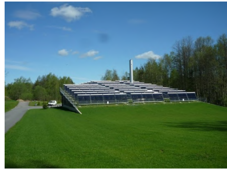
Figure 8.5. Installation of solar panels at the Pühajärve wood-fired district heating boiler house. (Photo Ü. Kask)
