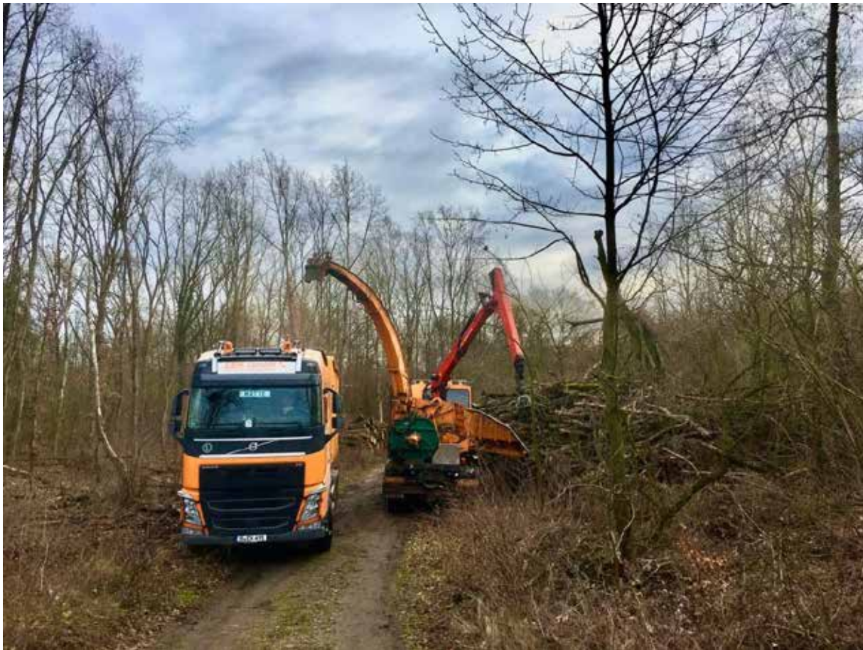
Picture 57. In Germany the capacity for chipping, transportation and storing of chips is available. (Photo: Mareike Schultze)
