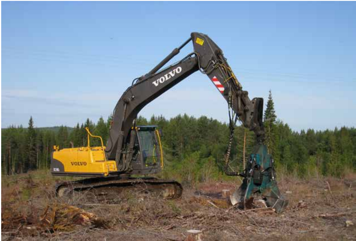
Picture 39. A heavy excavator is stable and strong enough for stump lifting. (Photo: Juha Laitila)
