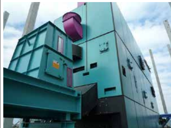
Picture 6. AS Kuressaare Soojus new combined heat and power plant. F
