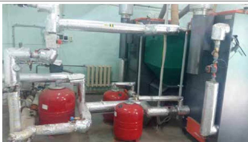
Picture 5. Boiler. (Photo: Valda Gudynaitė-Franckevičienė)
