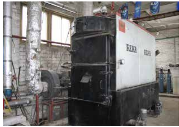
Picture 8. Reka boiler in Muhu Liiva boiler house.
